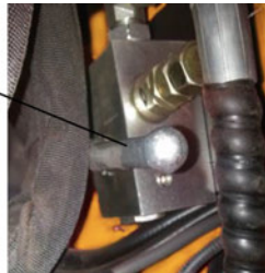
Three-way valve to horizontal position (ON)
